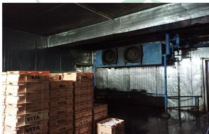
Storage at dairy product industries
