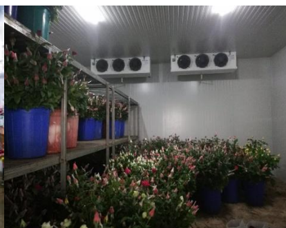
Flower cold storage room at Ghaziabad
