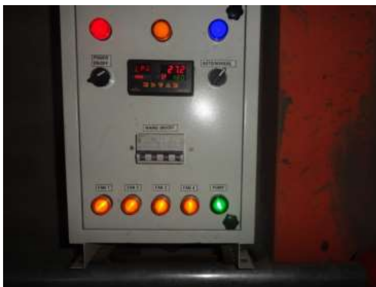
Automatic Temperature control unit
